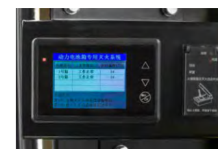
Automatic battery fire extinguishing devices
