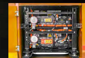
Battery and motor radiator
